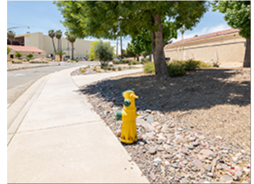
Standard Fire Hydrant
