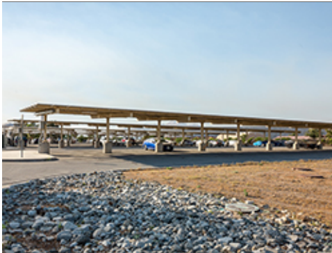
Photovoltaic (PV) Array Generating Electricity
