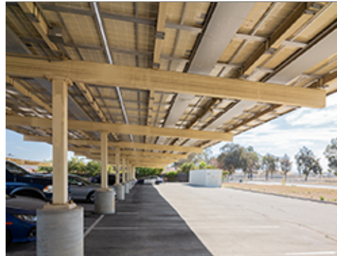
PV Array Providing Shading
