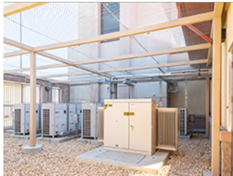
Service Cabinet in Visually Screened Yard
