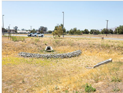
Detention Pond with Erosion Element
