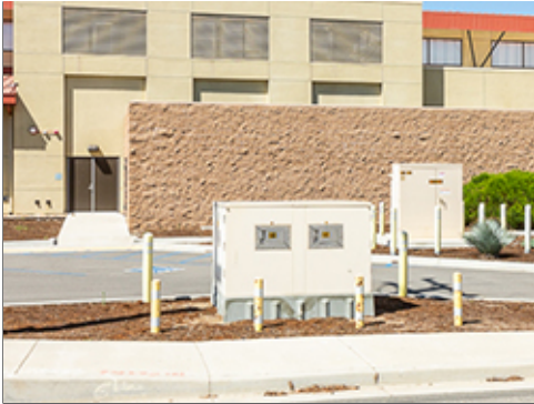
Electrical Cabinet at Roadway
