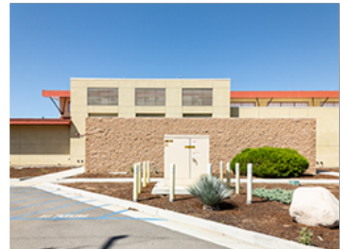
Ground Mounted Electric Cabinet
