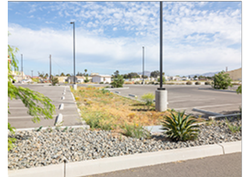
Bioswale for Rainwater Retention
