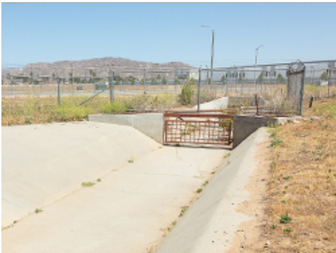
Channel with Debris Gate
