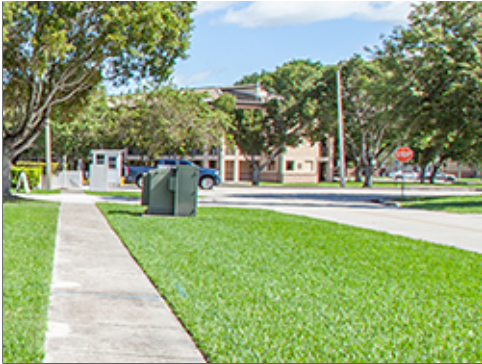
Unobtrusive Cabinet Location and Color
