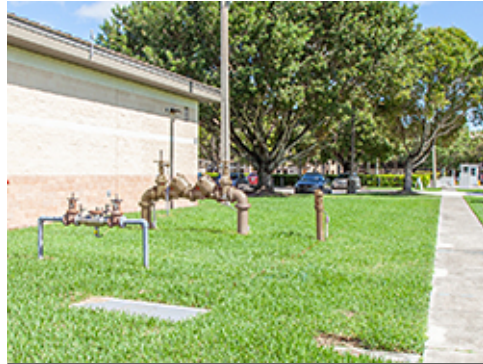
Inconspicuous Plumbing Elements
