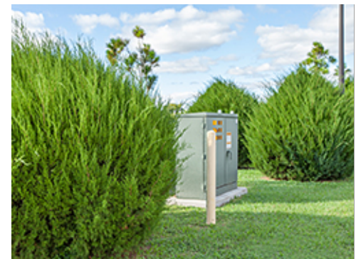
Landscape Screening of Cabinet
