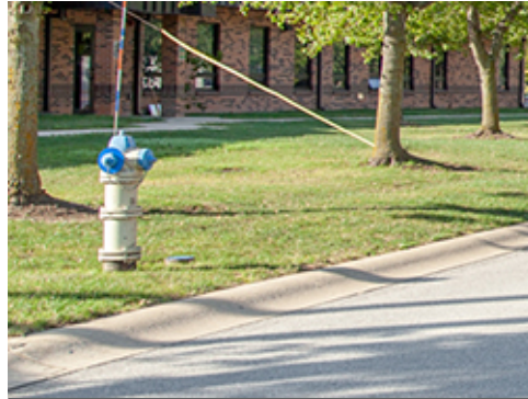
Typical Hydrant Location
