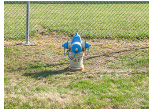
Base Standard Fire Hydrant
