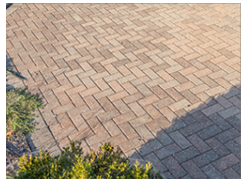
Concrete Pavers with Herringbone Pattern
