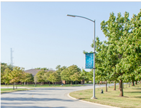
Street Fixture with Extended Arm
