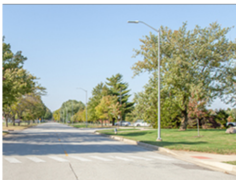
Typical Pole and Fixture
