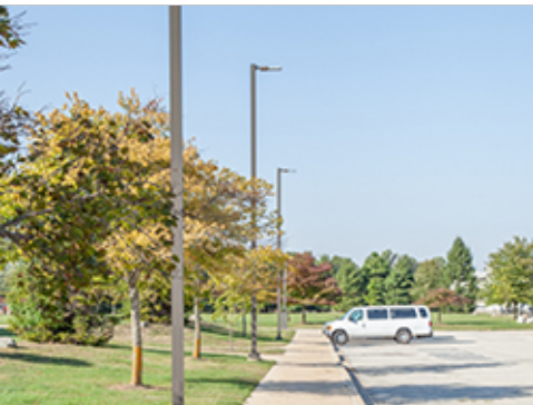
Combined Parking and Pedestrian Lighting
