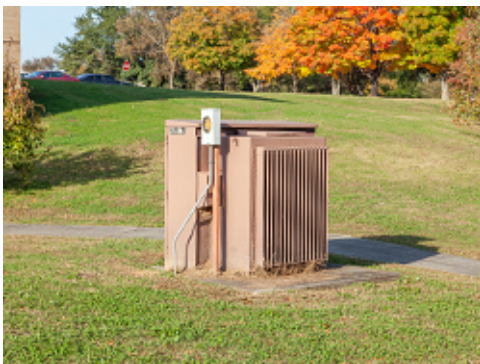
Standard Color for Electrical Transformer
