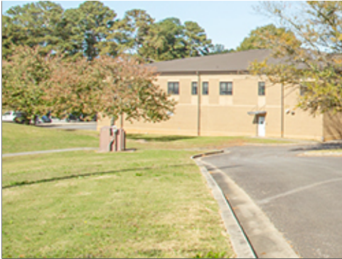
Electrical Transformer near Street
