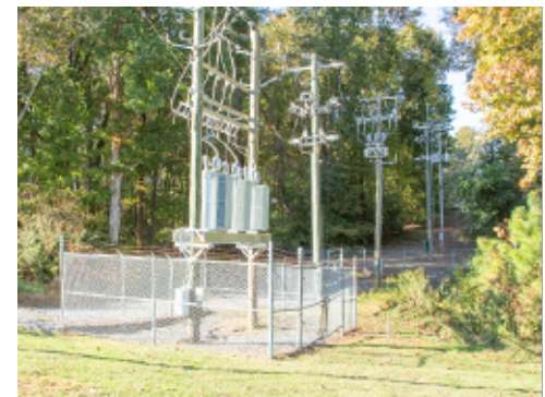
Fencing at Electric Substation
