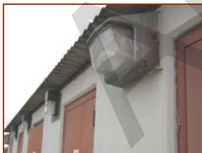
Figure 3.18 Security Lighting on Segregated Magazine - Langley AFB, VA
