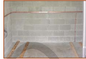
Figure 3.16 Grounding System Inside Flight Line Holding Facility - McChord AFB, WA
