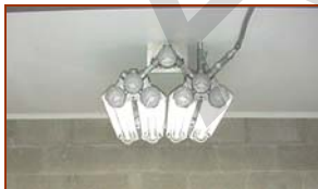
Figure 3.15 Explosive-proof Lighting in Flight Line Holding Facility - McChord AFB, WA
