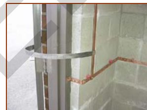
Figure 3.10 Grounding System Inside Flight Line Holding Facility - McChord AFB, WA
