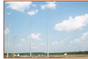
Figure 3.9 LPS (Catenary System) – Integrated Maintenance Facility - Barksdale AFB, LA
