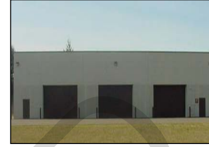
Roll-up Bay Doors with Personnel Entrances at Both Ends
