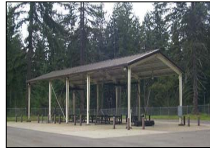
Munitions Assembly Conveyor (MAC) Pad
