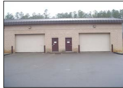
Facility Provides Good Security Lighting and Personnel Doors Adjacent to Roll-up Doors
