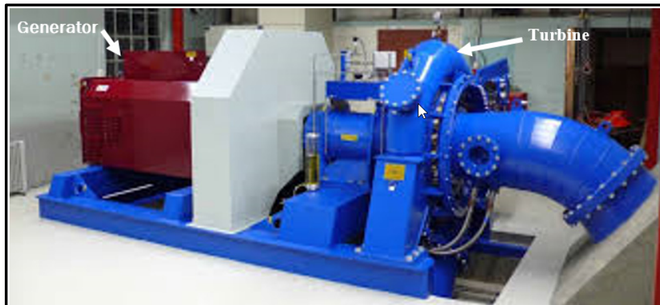
Figure 2. Skid mounted Francis turbine.
