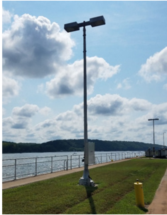
Figure 16. L&D No. 25, existing light fixtures.
