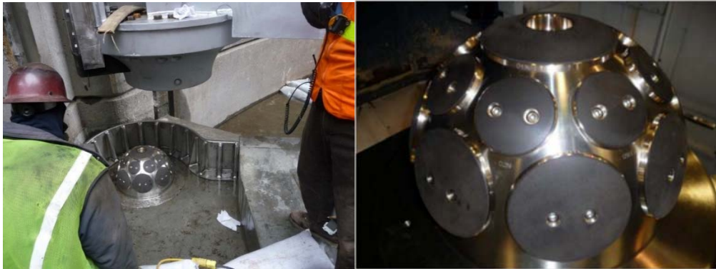
Figure 6. Miter gate self-lubricating pintle – The Dalles Lock and pintle puck system (USACE).
