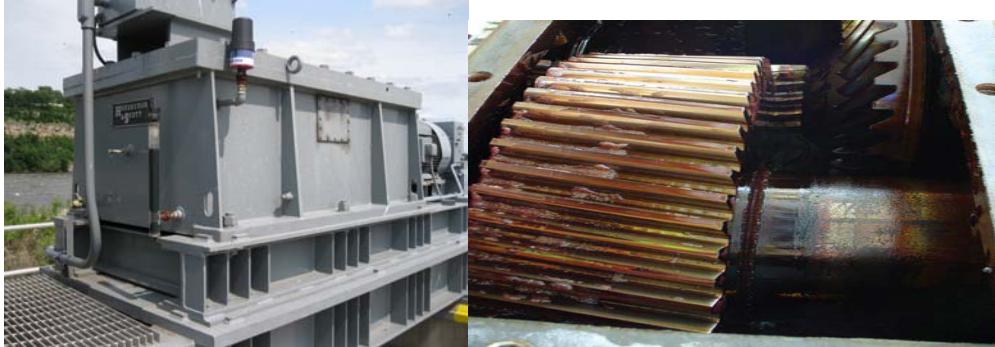
Figure 11. Gear reducers (USACE).
