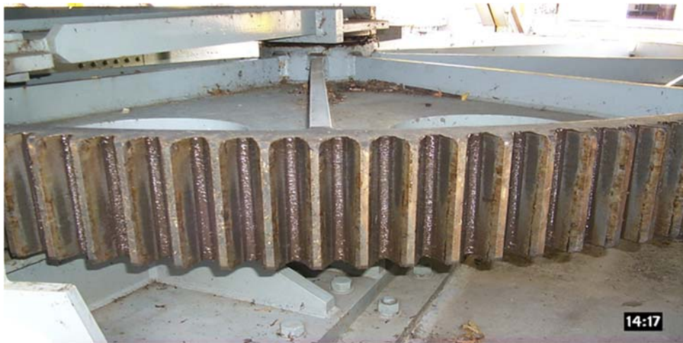
Figure 10. Sector gear (USACE).
