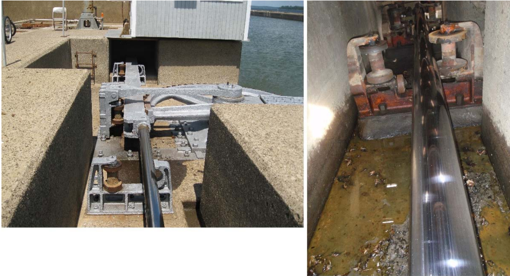
Figure 2. Lock 53 and LaGrange Lock hydraulic cylinders.
