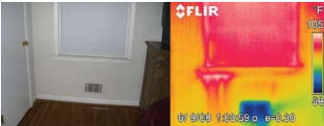
Figure 4. Air leakage is evident around a typical window. The leakage path appeared to be between the trim and the wall surface.
