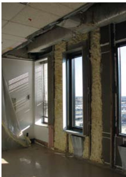
Figure 5. In-situ mockup of spray foam vs. rigid board insulation retrofit alternatives to validate design assumptions.
