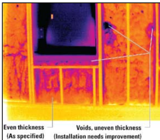
Figure 8. Thermal imaging part-way through the reinstallation of the insulation provided the Construction Manager information on what must be improved to meet the design specifications.
